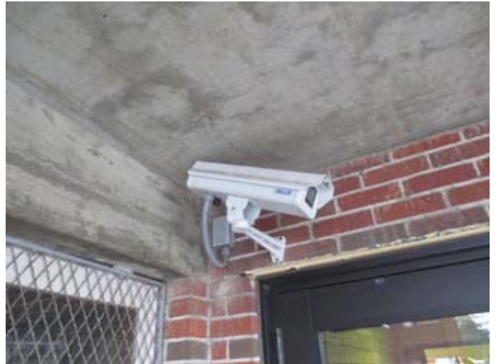
Exterior Security Camera
