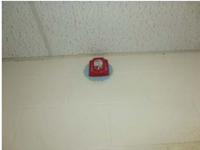
Fire Alarm Device
