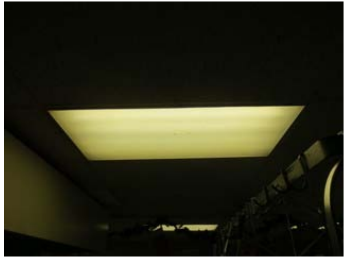
Kitchen Lighting Fixture
