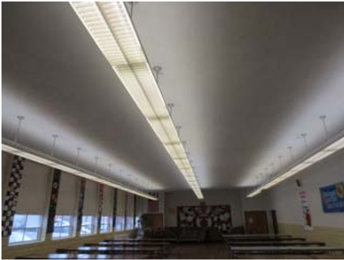
Student Dining Lighting Fixtures
