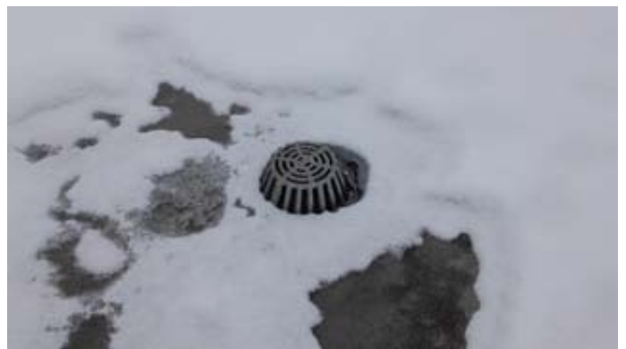
Typical Roof Drain
