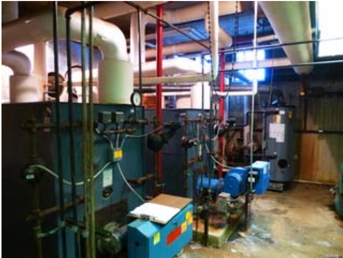
Existing Steam Boilers
