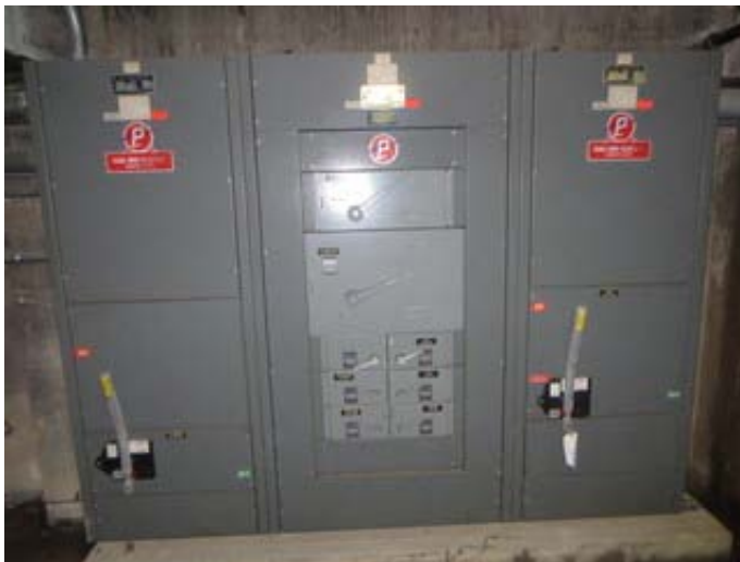
Main Electric Distribution
