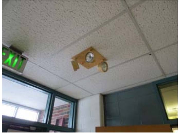
Emergency Egress Lighting Fixture
