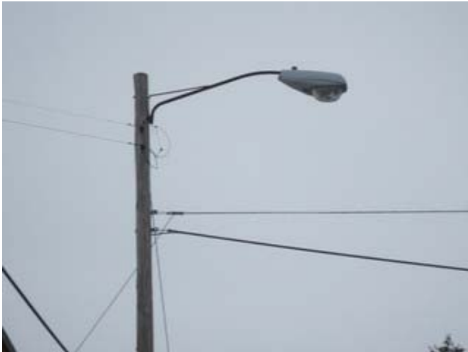
Site Lighting Fixture
