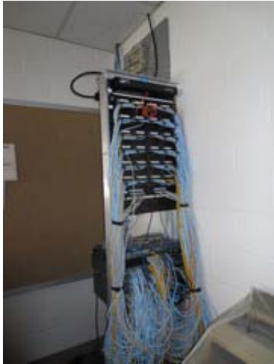
Data Main Distribution Rack
