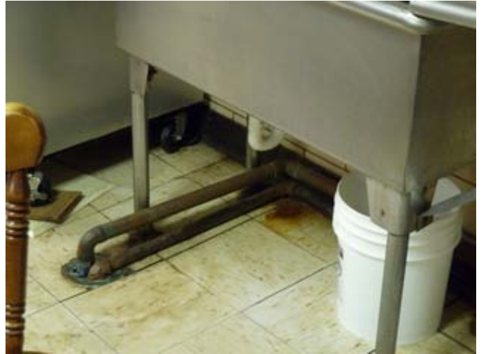
Kitchen Floor Drain
