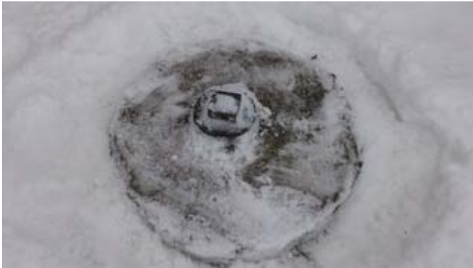
Exterior Clean Out
