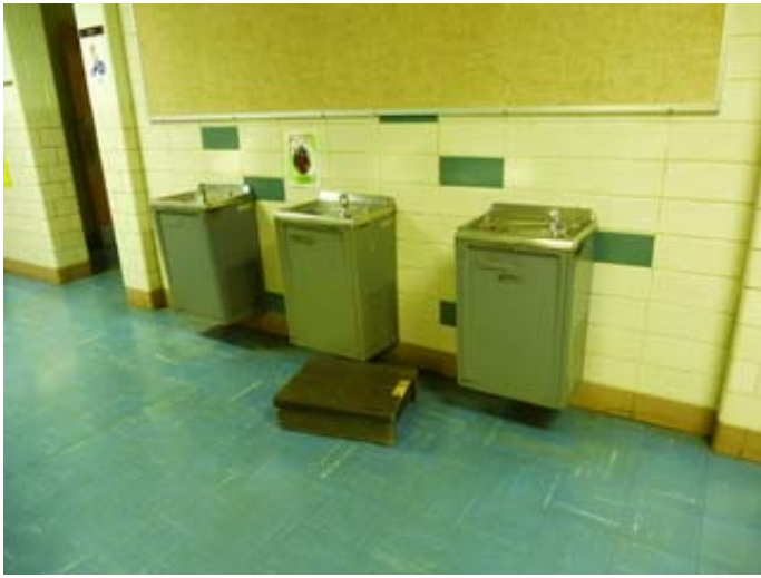
Typical Drinking Fountain
