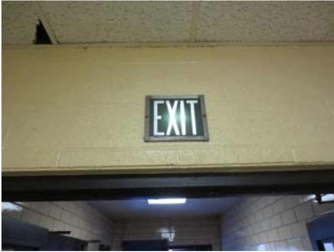
Incandescent Exit Sign
