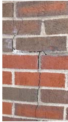
Cracking due to Insufficient Control Joints
