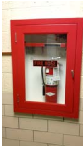
Fire Extinguisher Cabinet
