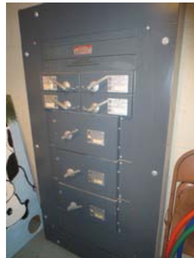
Addition Electrical Distribution
