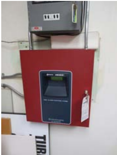
Fire Alarm Panel
