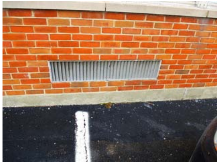
Unit Ventilator Outdoor Louver
