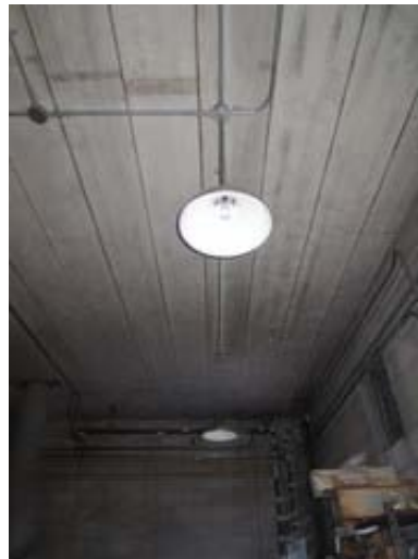
Service Area Incandescent Lighting Fixture
