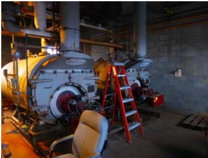
Existing Boiler Plant
