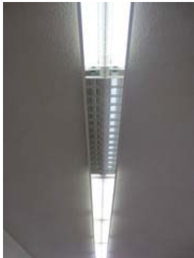
Classroom Lighting Fixture
