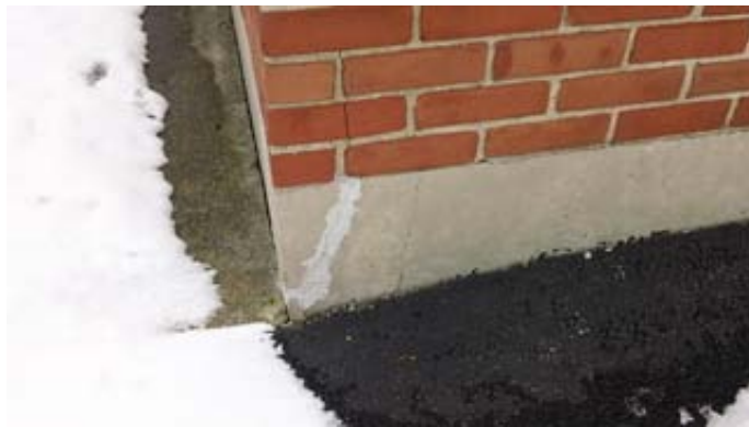
Damaged Concrete Foundation
