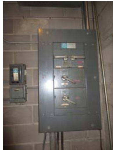
Original Electrical Distribution Equipment
