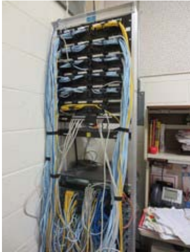
Main Data Distribution Rack
