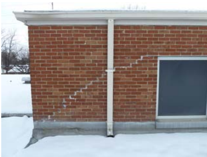
Exterior Masonry Wall Damage
