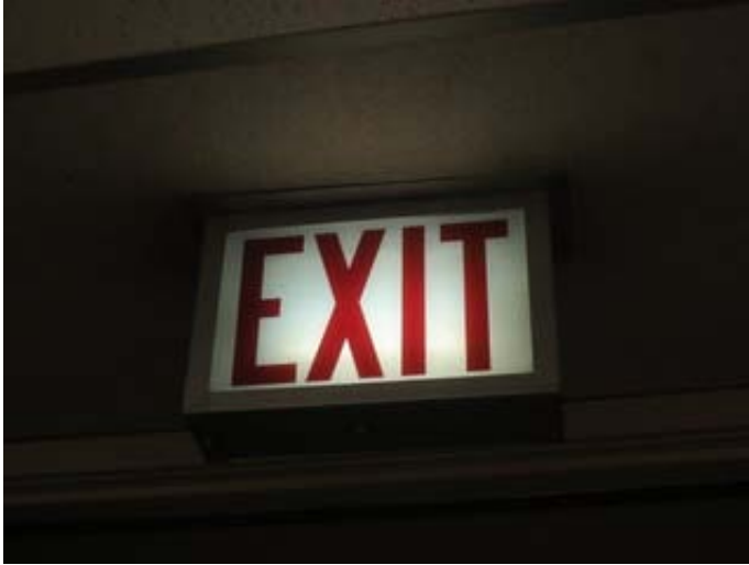
Non-Compliant Exit Sign
