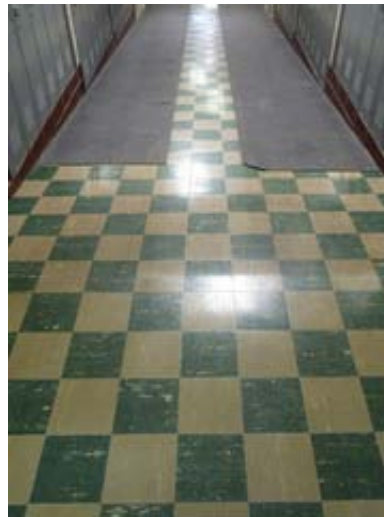
Existing Corridor Ramp without Handrails
