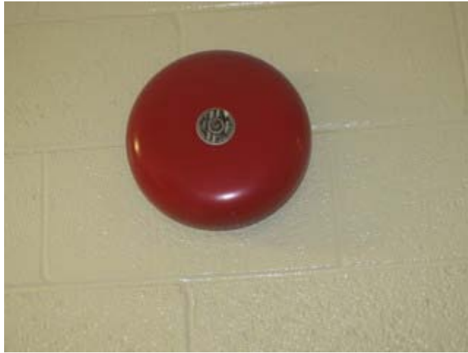
Fire Alarm Bell
