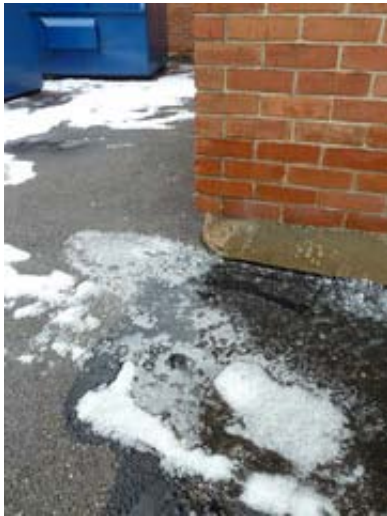
Deteriorated Concrete Foundation
