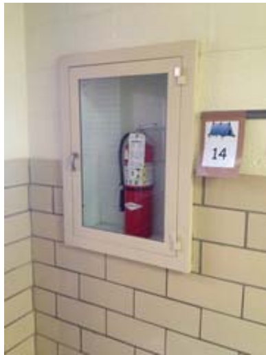
Recessed Fire Extinguisher
