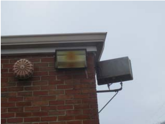
Exterior Site Lighting Fixtures
