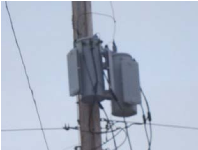
Utility Owned Transformer
