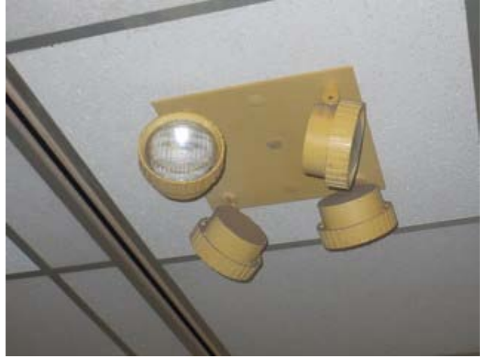
Emergency Egress Lighting Fixture
