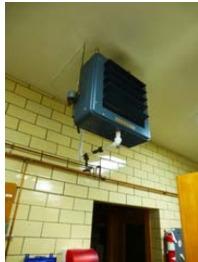
Existing Unit Heater
