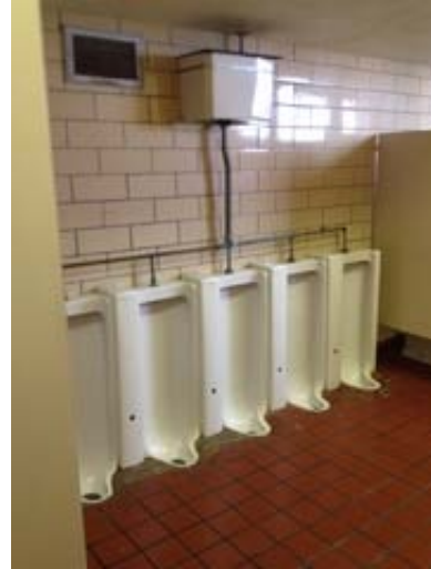
Urinals Double as Floor Drains
