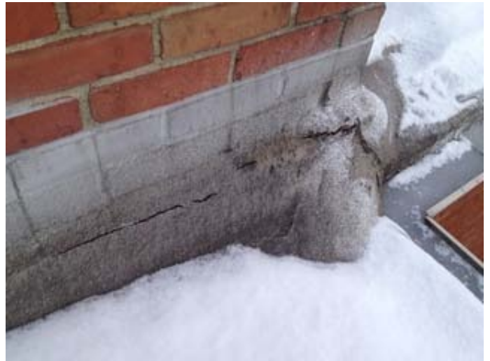
Roof Damage at a Corner Transition
