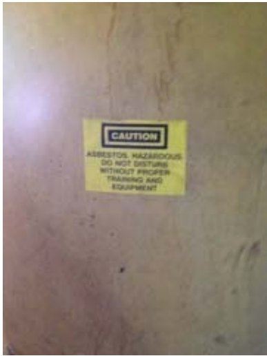
Water Tank Insulation
