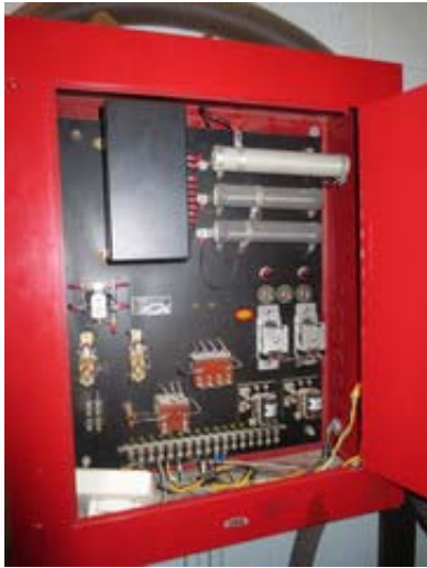
Fire Alarm Panel
