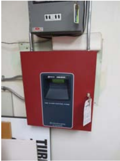
Broadway Elementary School Fire Alarm Panel
