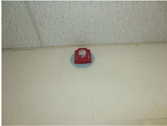
Fire Alarm Device
