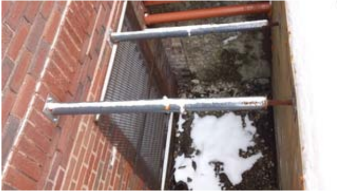
Failing Retaining Wall to Lower Level
