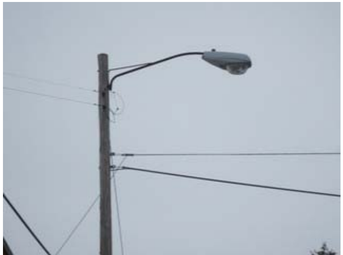
Exterior Site Lighting
