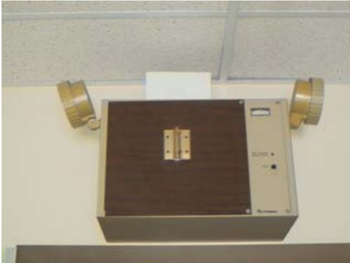
Emergency Egress Lighting Fixture
