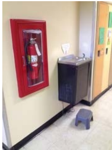
Fire Extinguisher Cabinet
