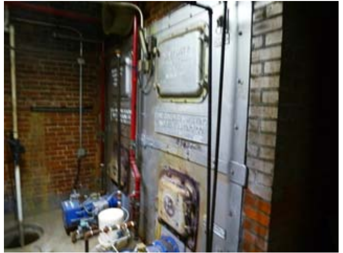
Gas Fired Forced Air Unit
