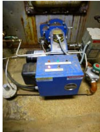
Existing Gas Burner
