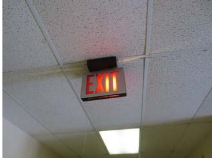
Incandescent Exit Sign
