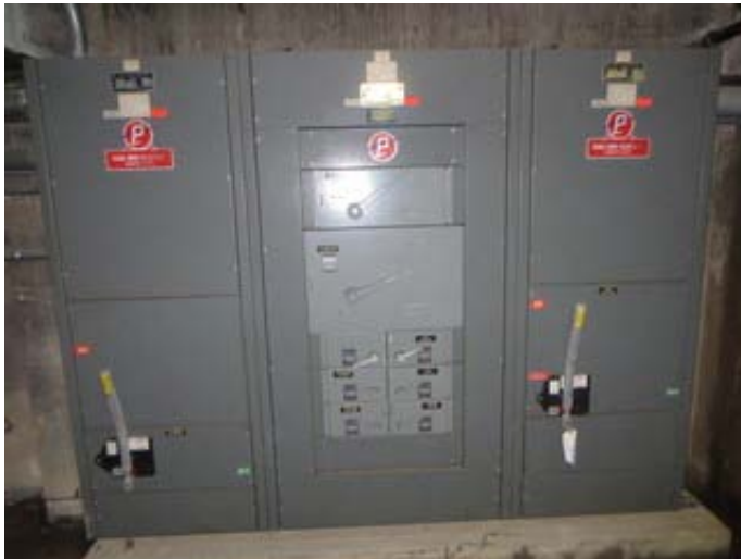
Broadway Elementary Gear that Provides Distribution
