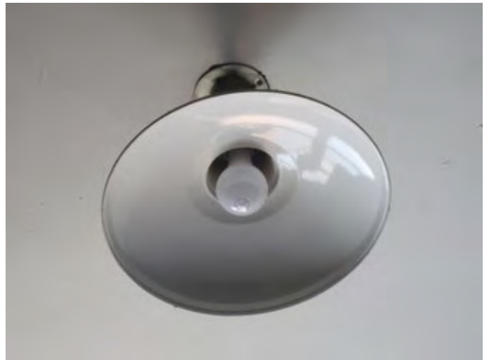
Service Area Incandescent Lighting Fixture
