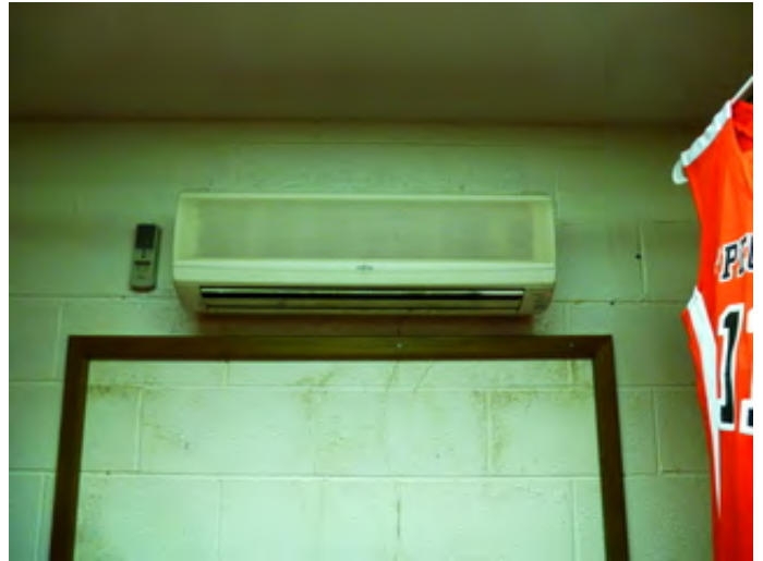
Existing Ductless Split System
