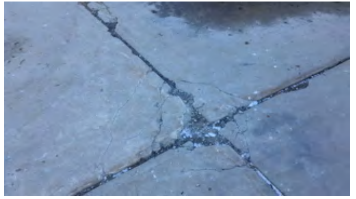
Typical Concrete Damage at the West Elevation Entry
