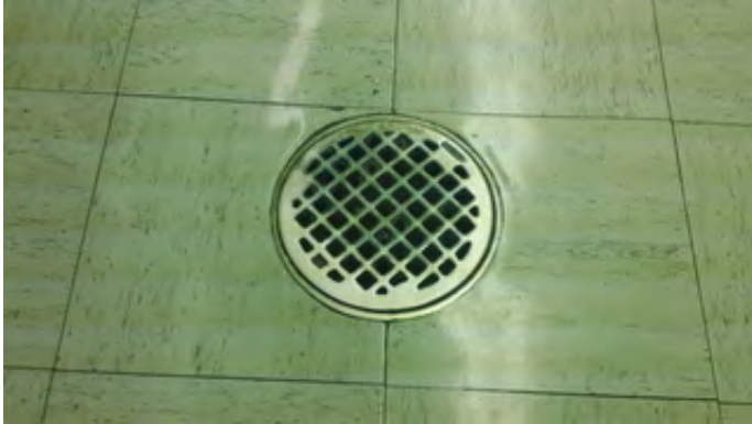
Kitchen Floor Drain
