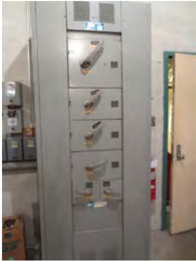
Electrical Distribution Equipment
