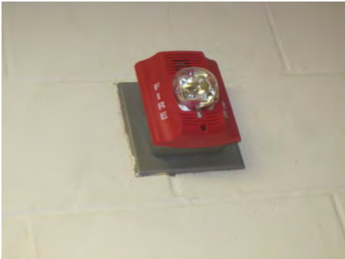
Fire Alarm Device
