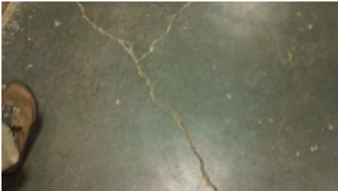
Locker Room Exposed Concrete Flooring Cracking
