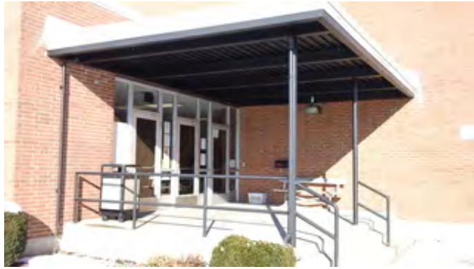
Inaccessible Main Entry
