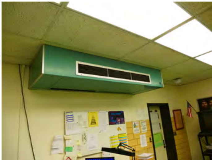
Existing Ceiling Mounted Unit Ventilator
