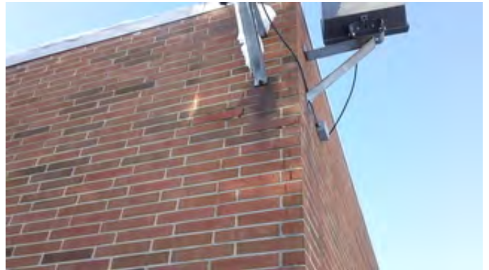
Corner Exterior Masonry Cracking
