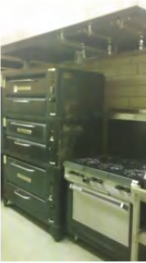
Kitchen Fire Suppression Hood
