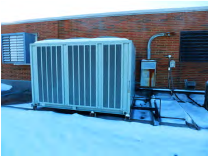
Existing Air Cooled Condensing Unit
