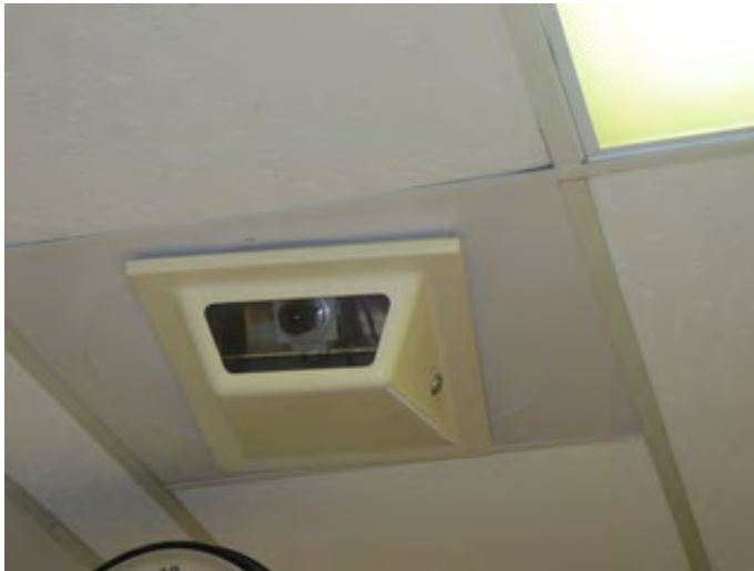
Inoperable Security Camera
