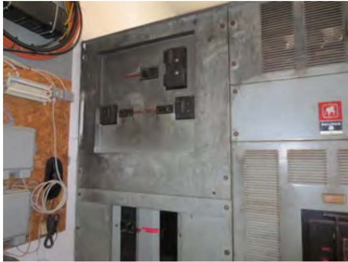
Main Electric Gear Smoke/Fire damage
