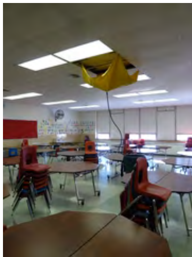
Student Dining Water Infiltration
