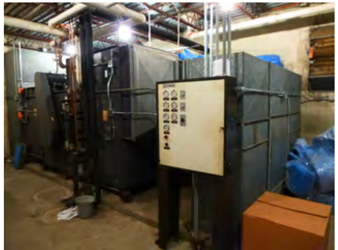
Existing Air Handler
