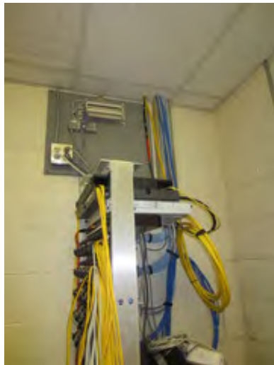
Main Data Distribution Rack
