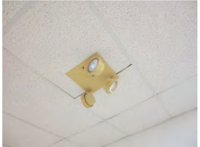
Emergency Egress Lighting Fixture
