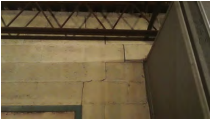
Damage Caused by a Lack of Control Joints
