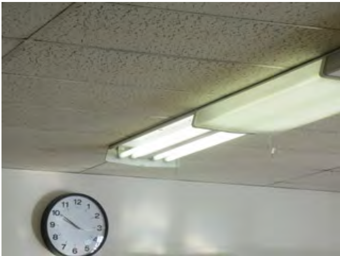
Classroom Lighting Fixture
