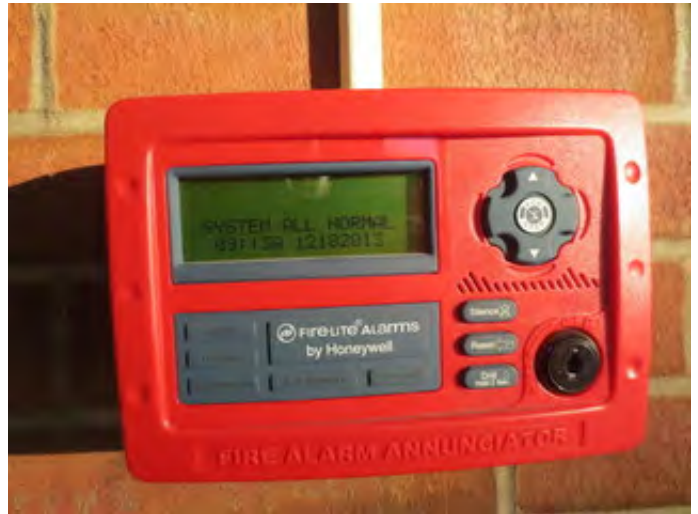
Fire Alarm Annunciator Panel
