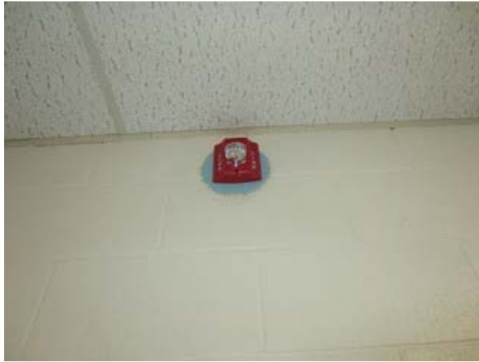
Fire Alarm Device
