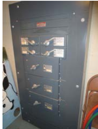
Addition Electrical Distribution
