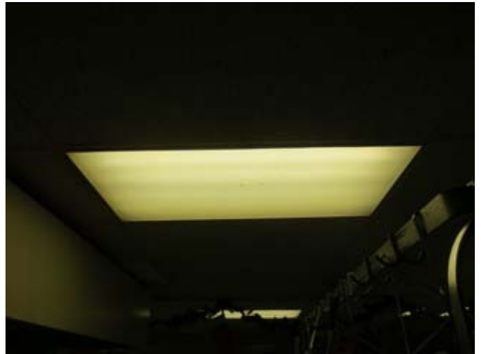
Kitchen Lighting Fixture
