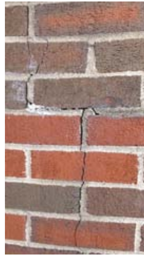
Cracking due to Insufficient Control Joints
