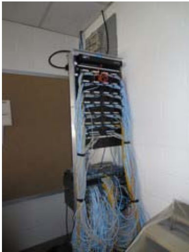
Data Main Distribution Rack
