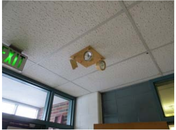
Emergency Egress Lighting Fixture
