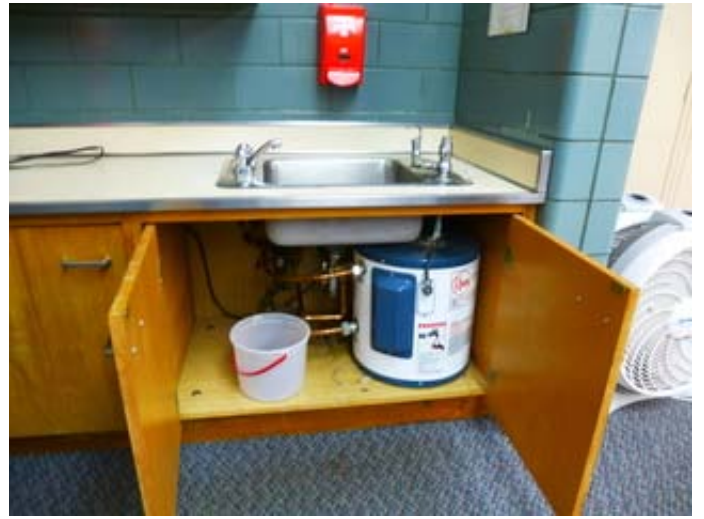
Under the Counter Water Heater
