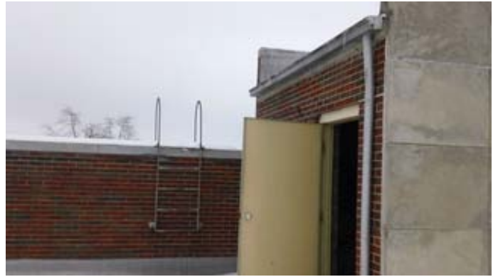
Roof Access Door
