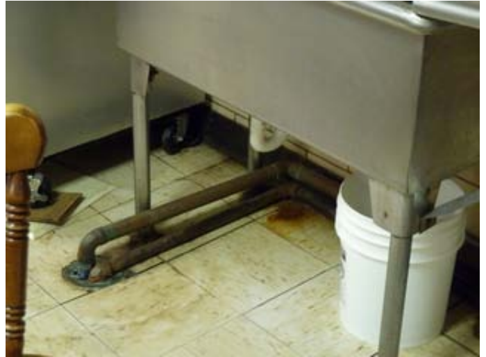
Kitchen Floor Drain
