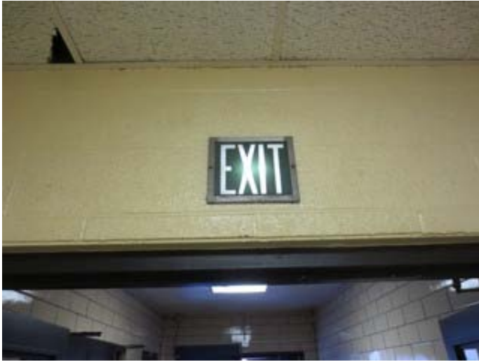
Incandescent Exit Sign
