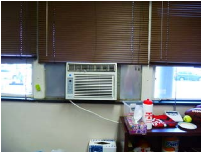
Typical Window A/C Unit
