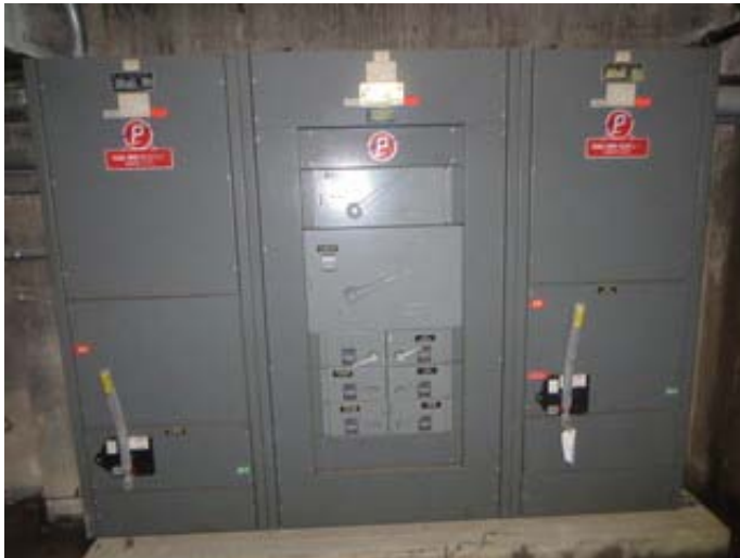
Main Electric Distribution
