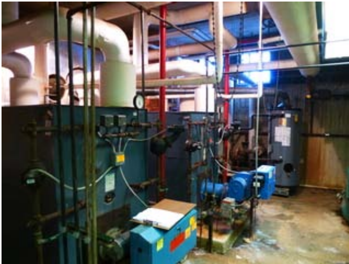
Existing Steam Boilers
