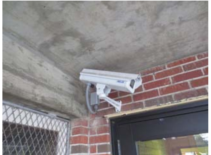
Exterior Security Camera
