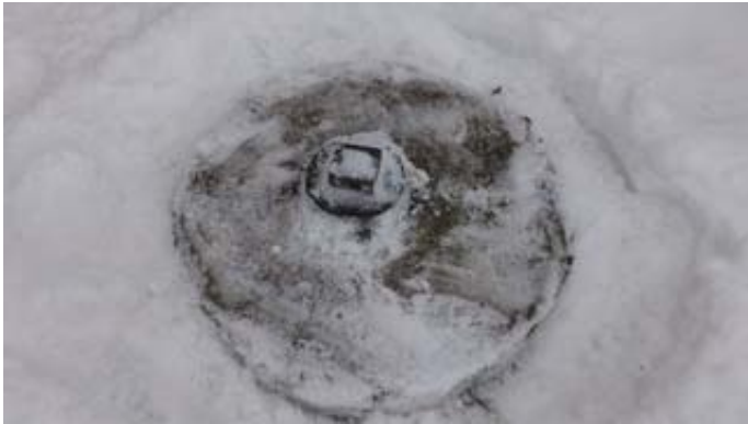
Exterior Clean Out
