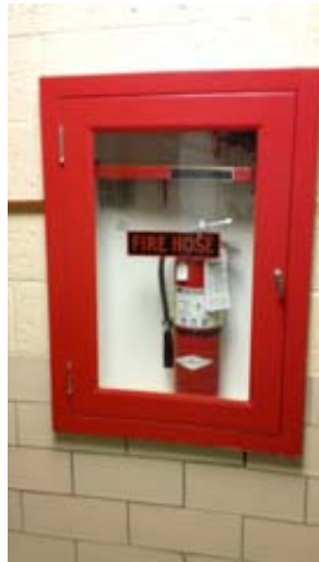
Fire Extinguisher Cabinet
