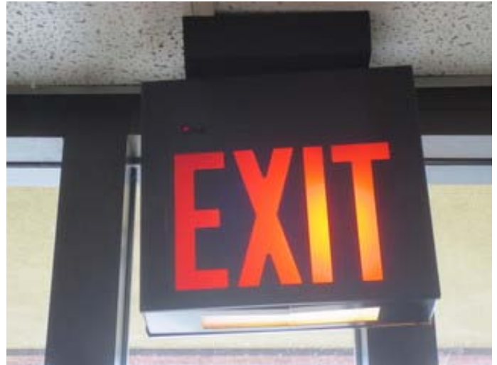
Non-Compliant Exit Sign
