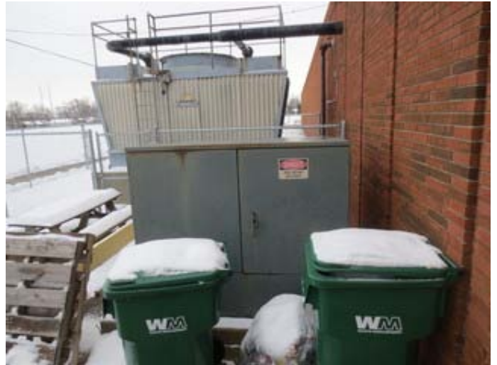
District Owned Transformer
