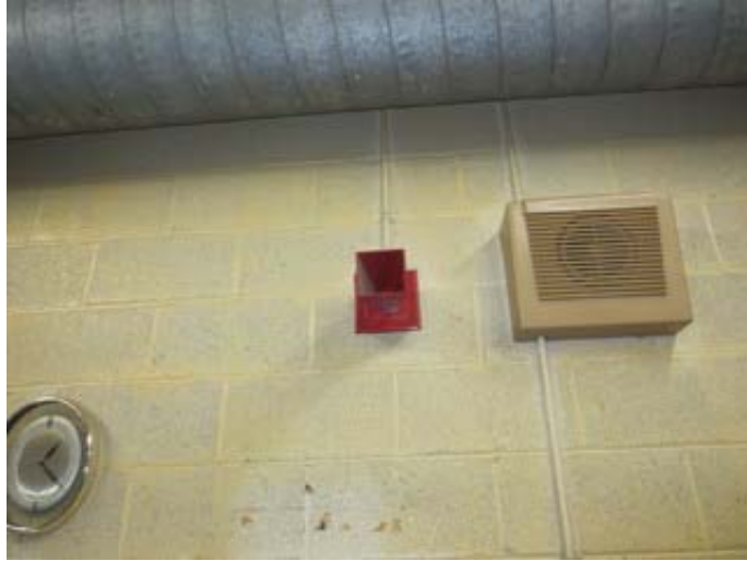
Fire Alarm Horn
