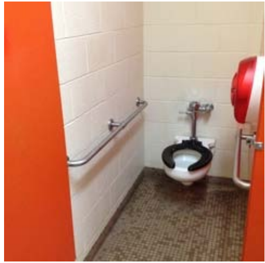
Typical Non-Compliant Stall Configuration
