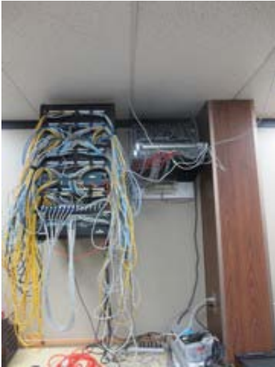
Main Data Distribution Rack
