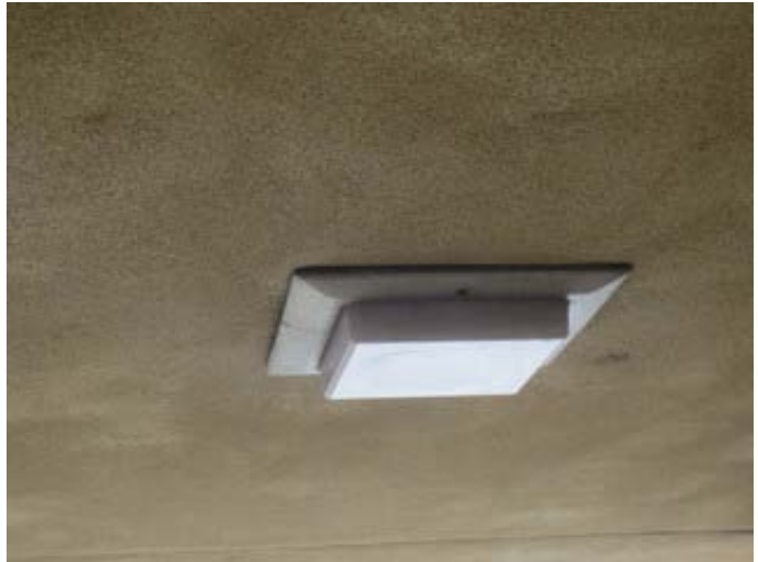
Entry Canopy Lighting Fixture
