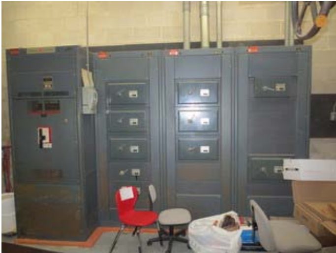
Main Electrical Gear
