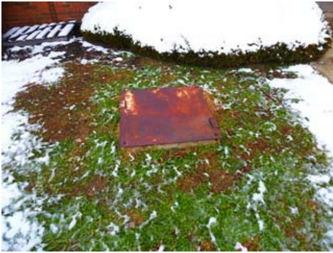
Existing Grease Interceptor
