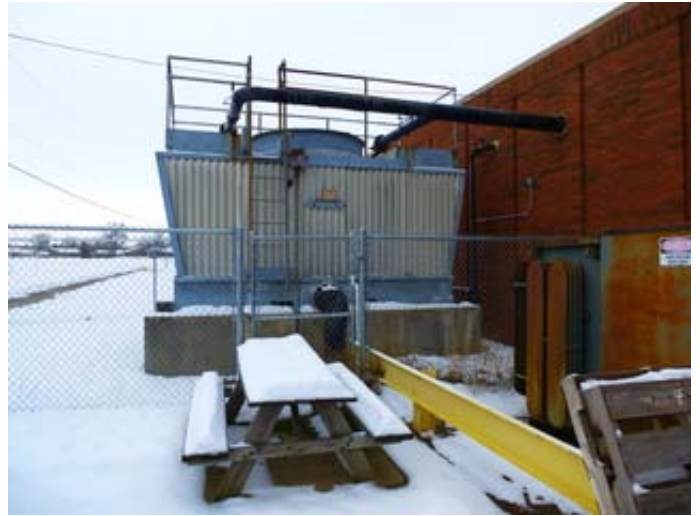
Existing Cooling Tower
