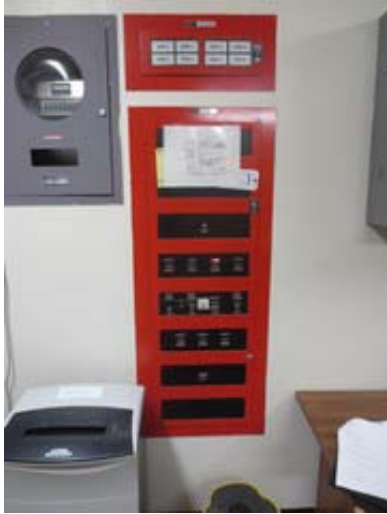
Fire Alarm Panel
