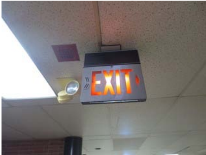
Exit Sign and Emergency Lighting Fixture
