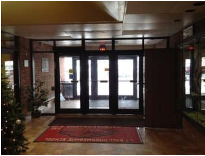
Power Assisted Main Entrance
