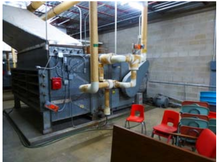
Existing Air Handler
