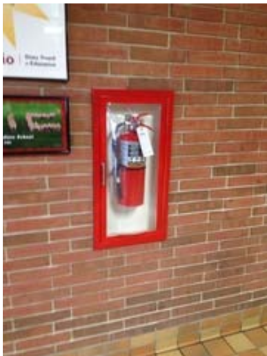
Typical Fire Extinguisher Cabinet
