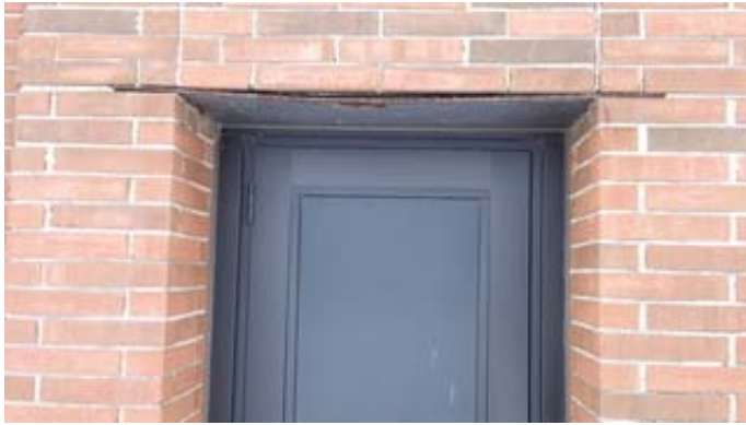
South Elevation Lintel Condition
