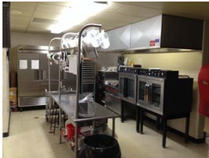
Exhaust Hood with Suppression System
