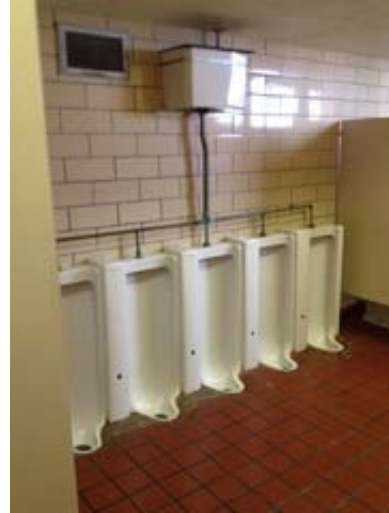
Urinals Double as Floor Drains
