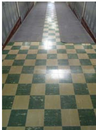
Existing Corridor Ramp without Handrails
