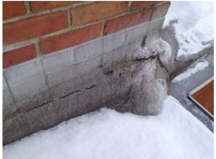
Roof Damage at a Corner Transition
