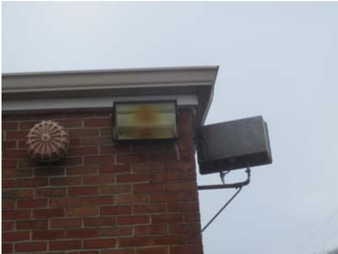
Exterior Site Lighting Fixtures
