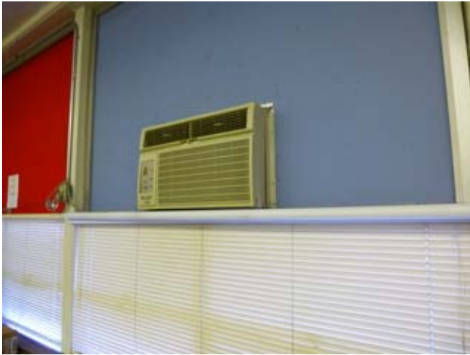
Typical Window A/C Unit
