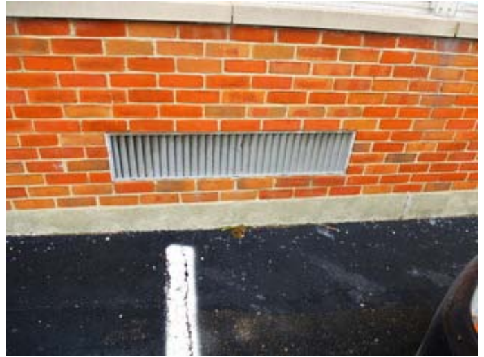
Unit Ventilator Outdoor Louver
