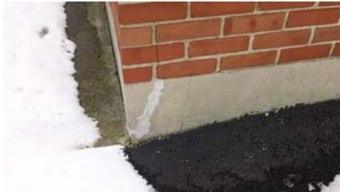
Damaged Concrete Foundation
