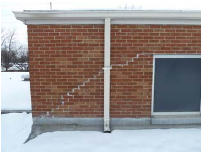
Exterior Masonry Wall Damage
