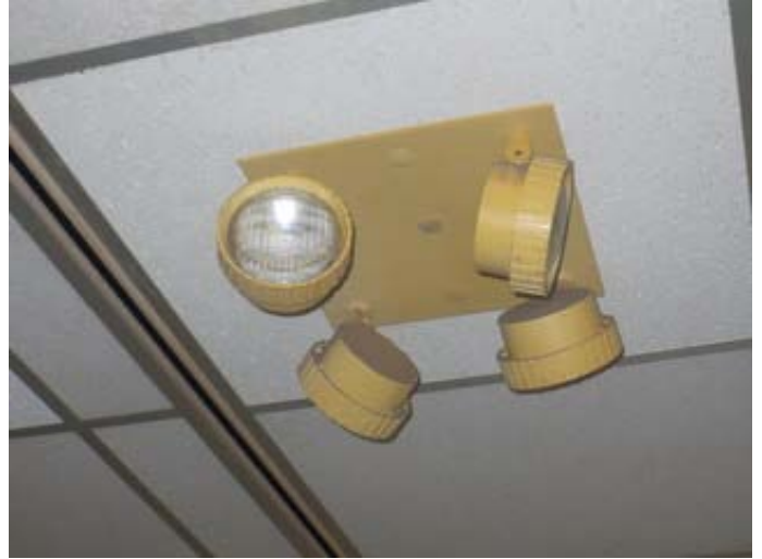
Emergency Egress Lighting Fixture
