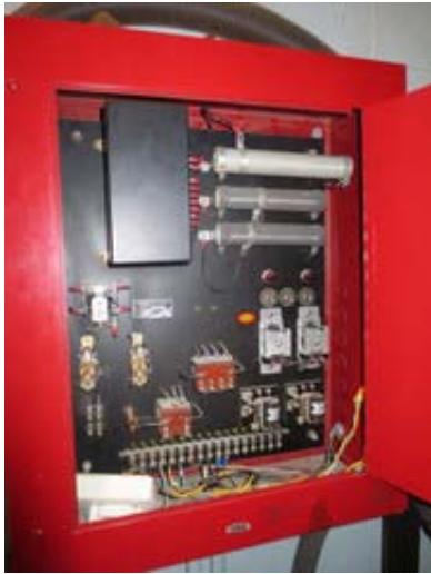
Fire Alarm Panel
