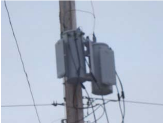
Utility Owned Transformer
