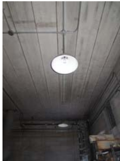
Service Area Incandescent Lighting Fixture
