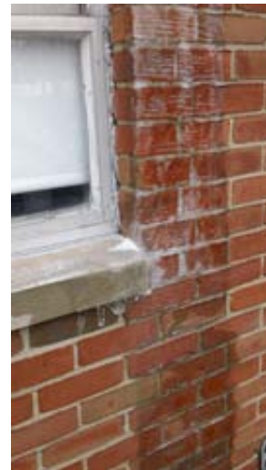
Ice Formation on the Facade Adjacent to a Window Unit
