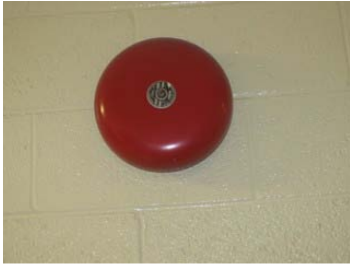
Fire Alarm Bell
