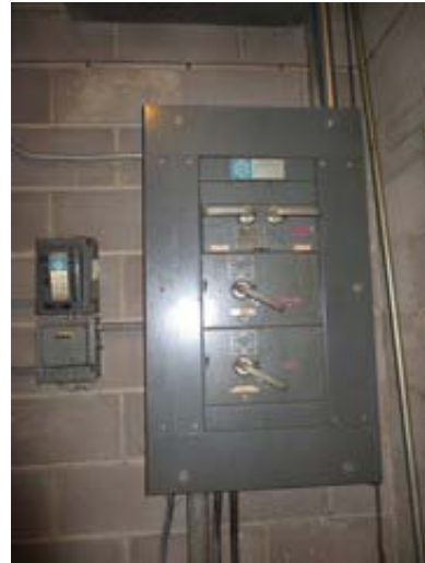
Original Electrical Distribution Equipment
