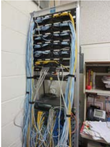
Main Data Distribution Rack
