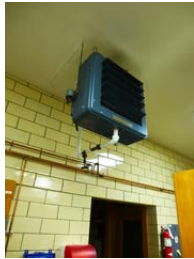
Existing Unit Heater
