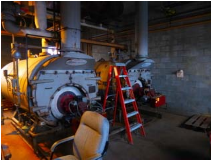
Existing Boiler Plant
