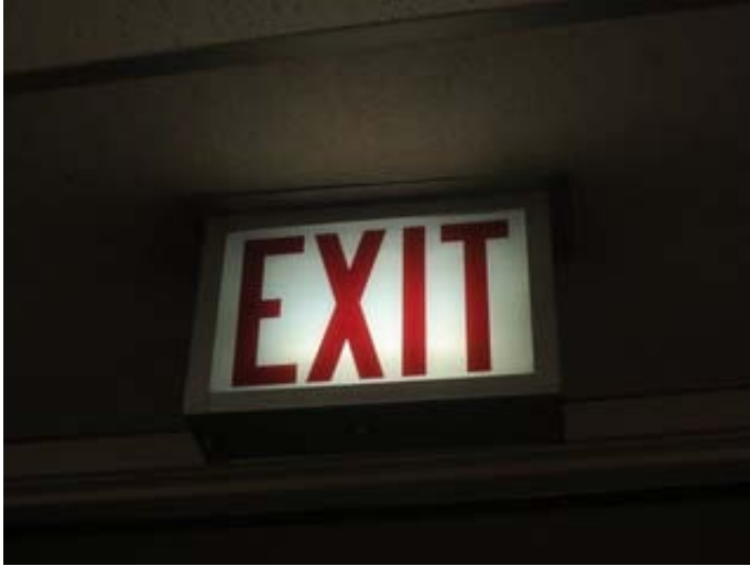
Non-Compliant Exit Sign
