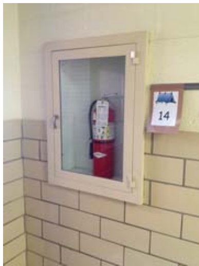
Recessed Fire Extinguisher
