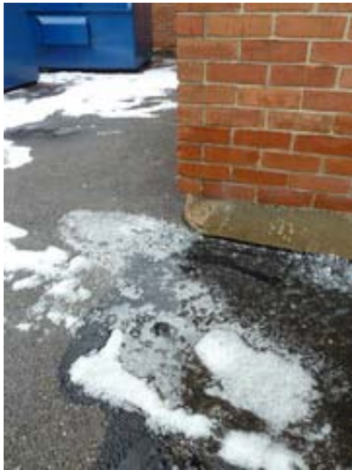
Deteriorated Concrete Foundation
