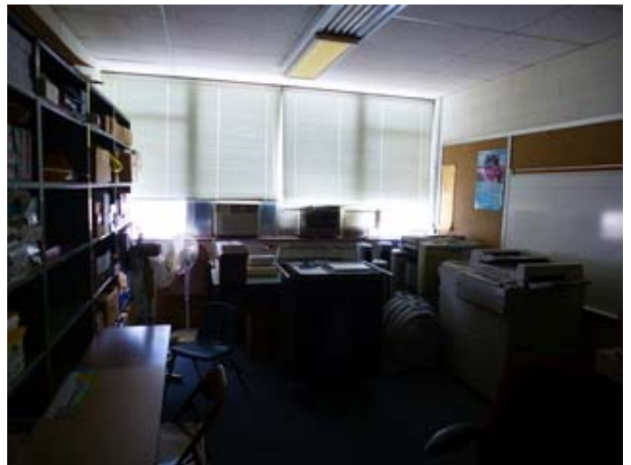
Storage Lighting Fixture
