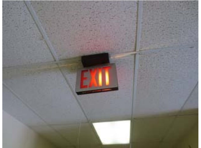
Incandescent Exit Sign
