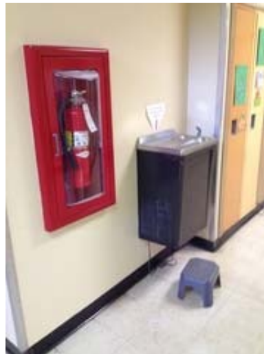
Fire Extinguisher Cabinet
