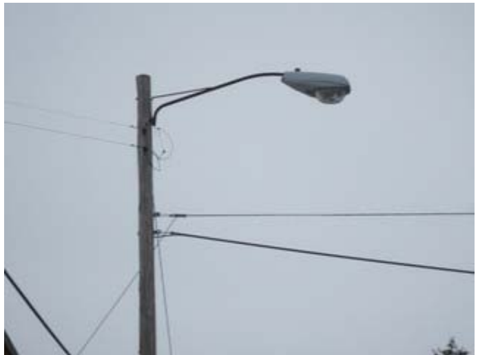
Exterior Site Lighting
