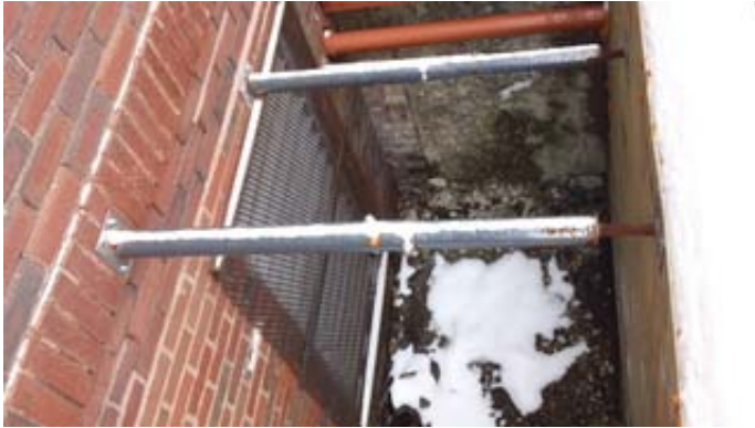
Failing Retaining Wall to Lower Level
