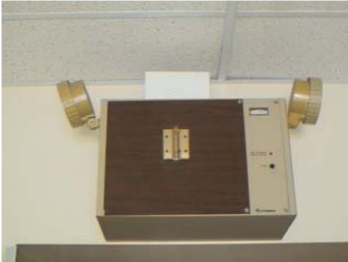
Emergency Egress Lighting Fixture
