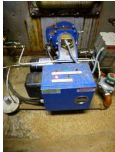
Existing Gas Burner
