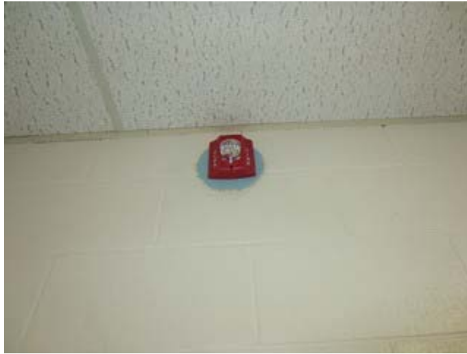
Fire Alarm Device
