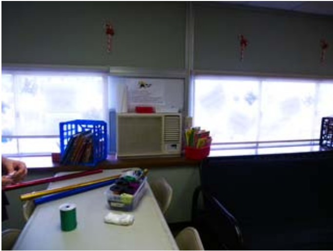
Typical Window A/C Unit
