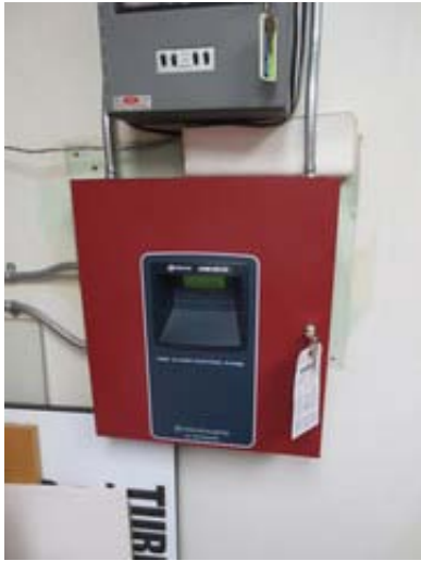
Broadway Elementary School Fire Alarm Panel
